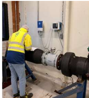
Figure: Zonal water meter
