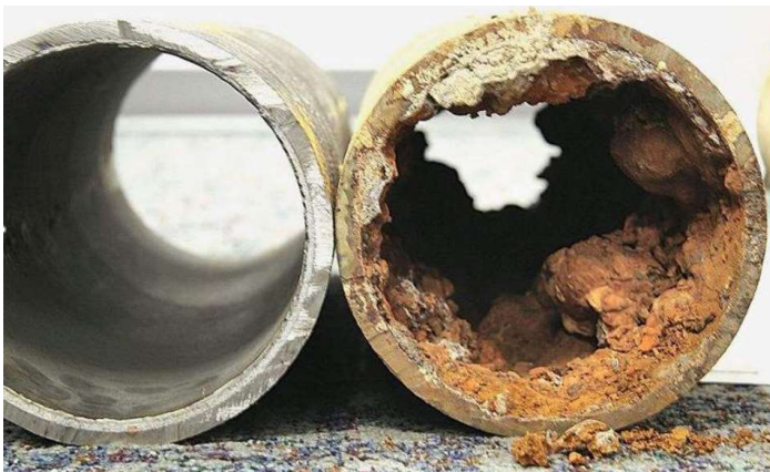
Photo: The wastewater pipe system is in bad shape, the capacity is diminishing
